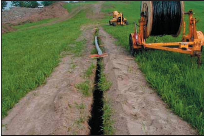
Electrical Line Interconnect
