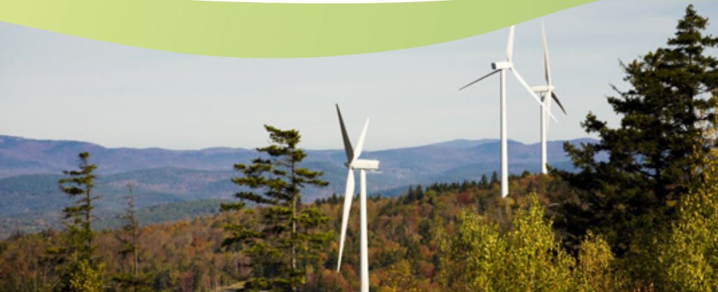
The Lempster Wind Farm in New Hampshire features 12 Gamesa G87 wind turbines that have a total capacity of 24 megawatts (MW).
