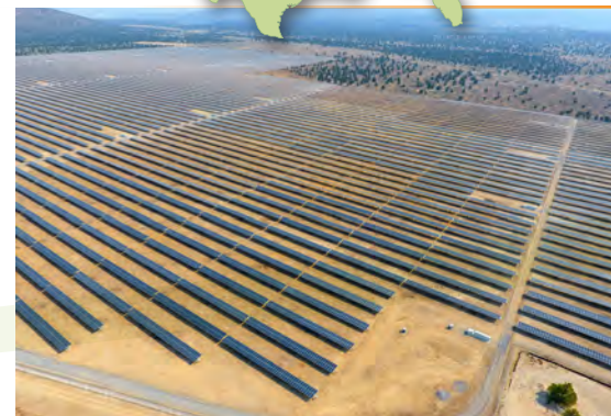
The 56 MW Gala Solar Plant, near Prineville, Oregon.
